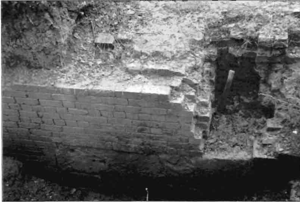
8. The southern plinth of Area 2, showing the partly undamaged inner face and the cut-off holding-down bolt still in situ .
